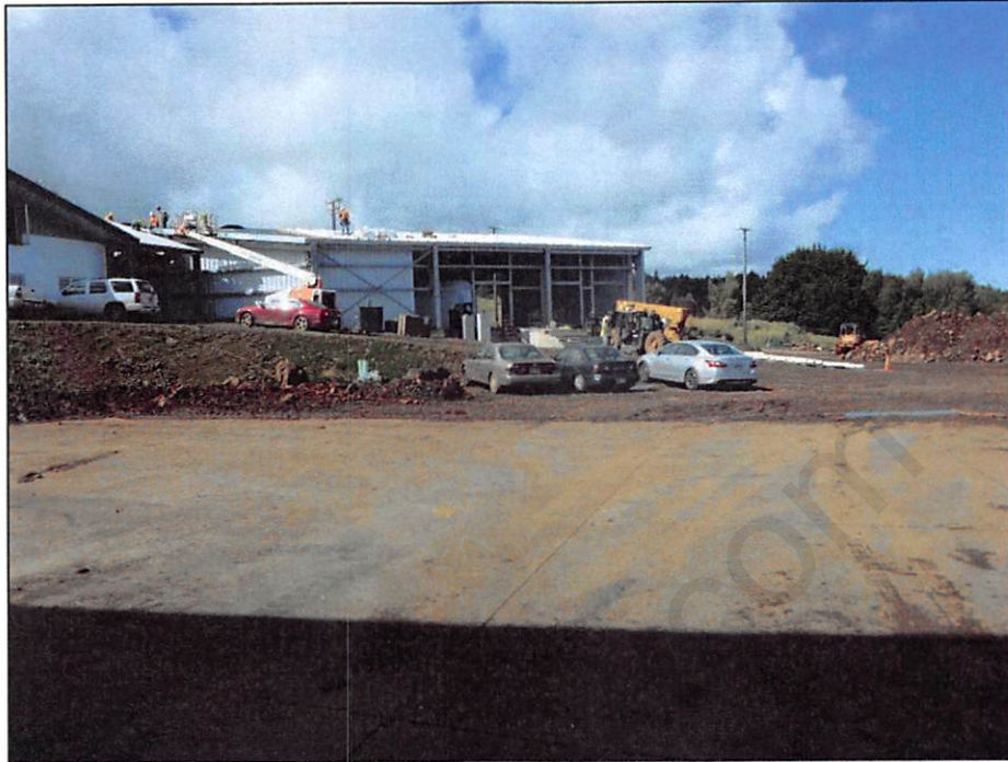
Photograph 3. View of the Facility's new building that was under construction at the time of the inspection. Photo by A. D'Angelo; 12/14/16.
