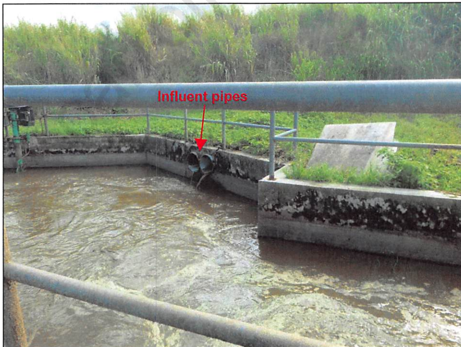
Photograph 16. View of the manure composting building collection pit influent pipes. Photo by A. D'Angelo; 12/14/16.
