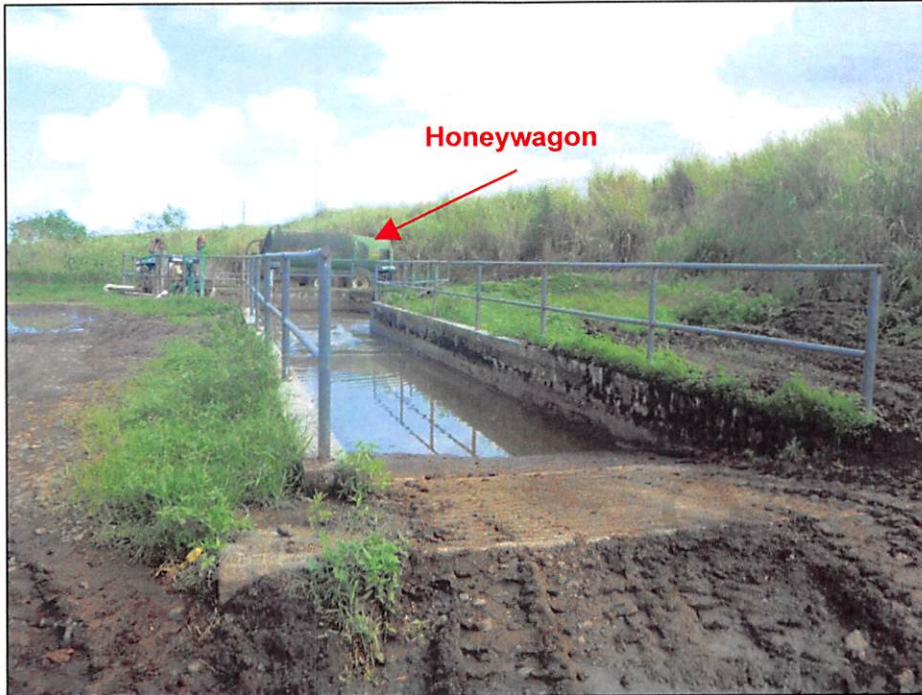
Photograph 15. View of the Facility's manure composting building collection pit. Waste streams from the freestall barns, calf barn, and milking barn gravity flow into this collection pit. Note the honeywagon stored behind the collection pit. Photo by A. D'Angelo; 12/14/16.
